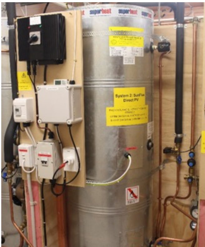
One of the 3 direct PV systems being assessed. It shows some of the complexity associated with the research setup. Where water temperature stratification, water and energy flows, and datalogging has to all be carried out in a controlled manner.
